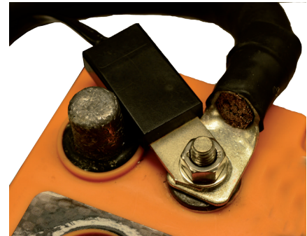
Fig 2.5(b) Temperature Sensor Installation
